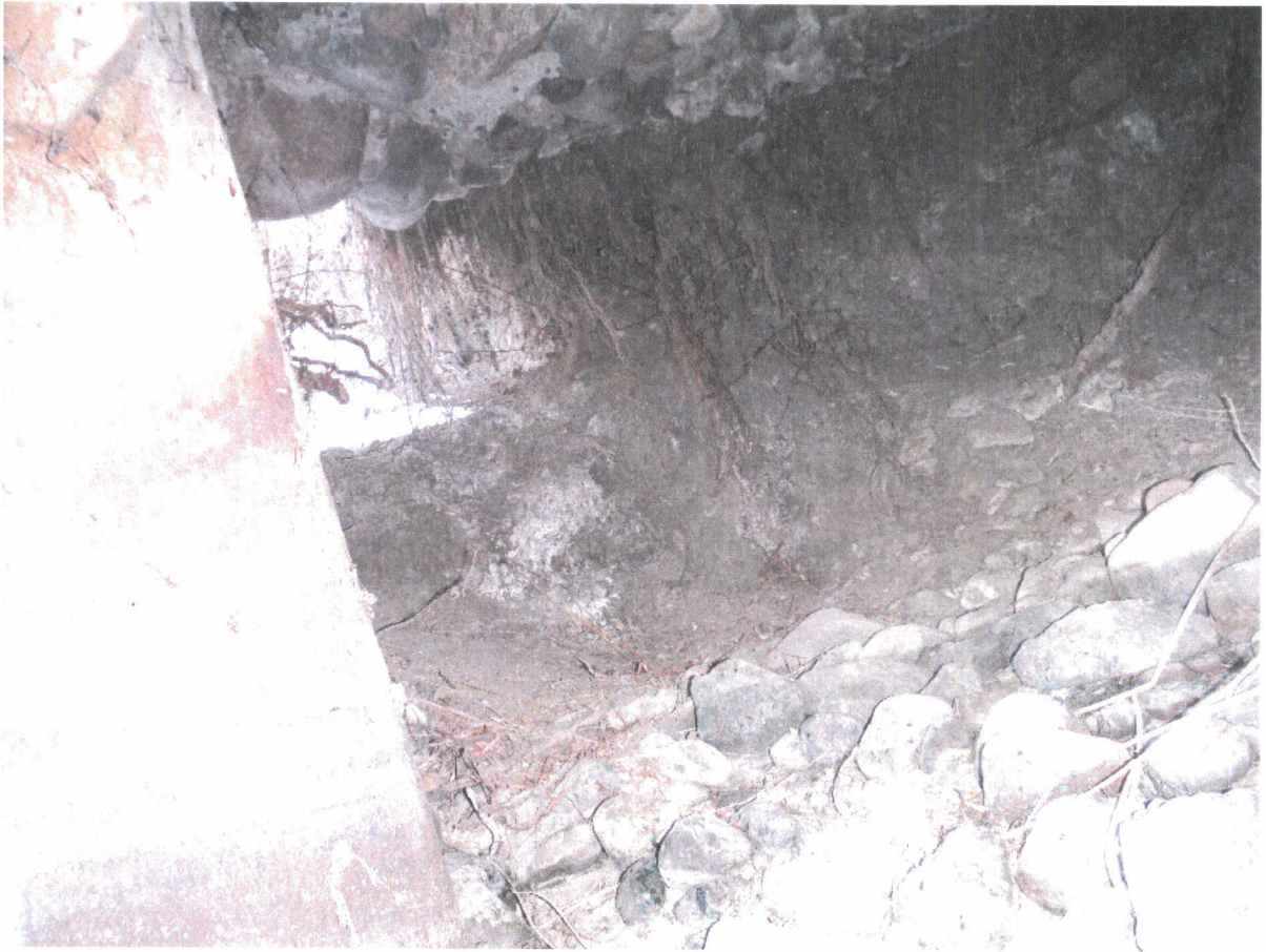
Figure 1: Erosion under spillway wingwall (daylight showing through on far side)
