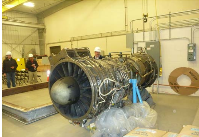
Figure 7: An example of the turbines used at the Dave Gates Generating Station.
