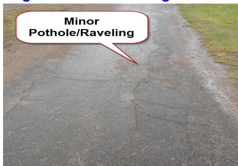
Figure Three: Raveling
