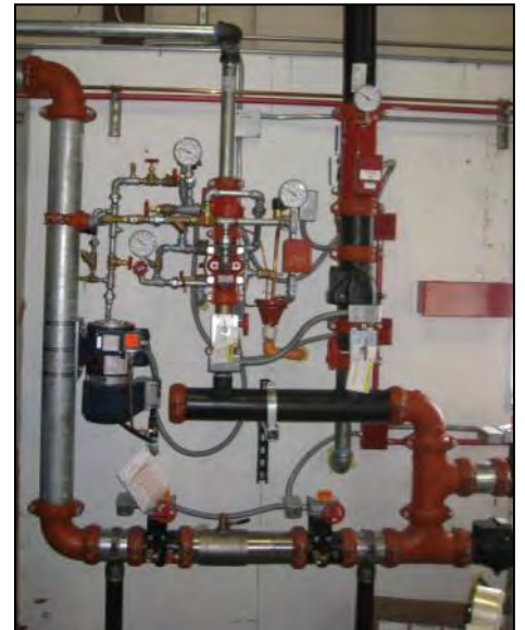
Prison maintenance upgraded the fire detection and protection system for the license plate factory.
