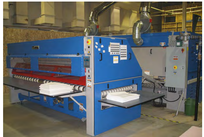
Energy efficient, commercial equipment was installed in the high-side laundry at MSP to handle all inmate clothing.
