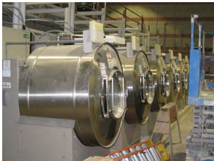
The energy efficient, commercial-sized equipment allows the new high-side laundry to handle all inmate clothing and creates new jobs for inmate workers.
