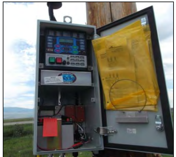
The new phase power protector installed at the prison replaces an unreliable old switch that allowed electrical equipment to be damaged.
