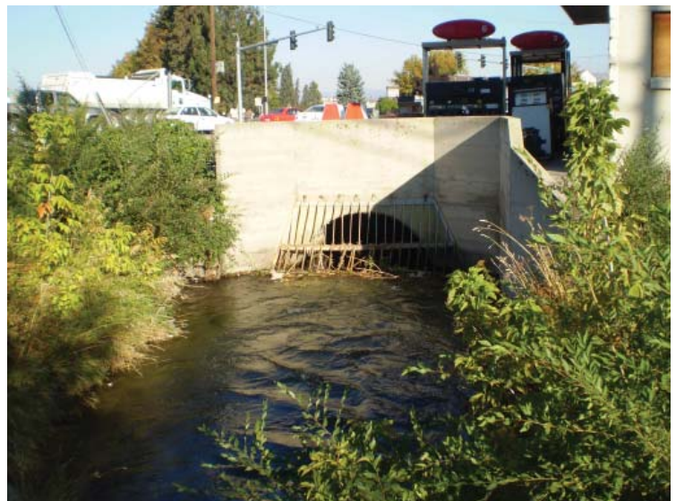
Urban Irrigation Canal, Grate for Safety and Trash Rack
