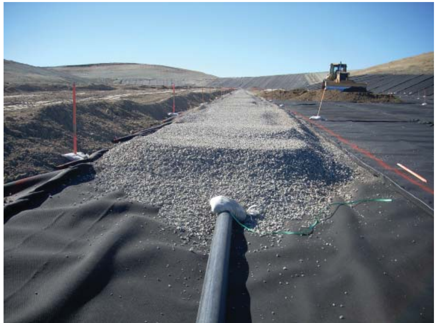
Gallatin County Landfill – Logan: Leachate Collection Trench
