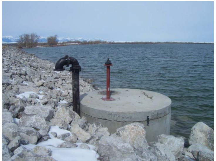
Newly constructed concrete outlet works for Teton County, Montana dam. The need for outlet replacement was identified during the engineer's inspection.
