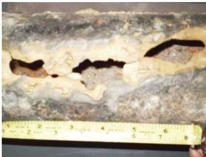
Corroded Cast Iron Water Pipe, 75-100 Years Old, Cascade, Montana
