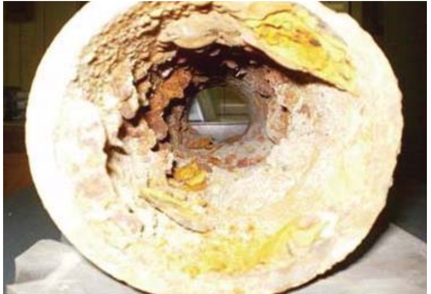
Corroded Cast Iron Water Pipe, 75-100 Years Old, Cascade, Montana
