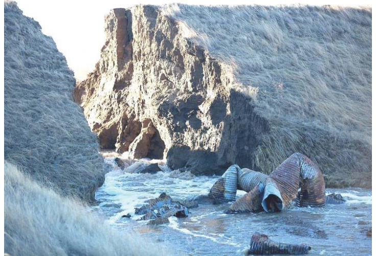
Recent failure of Choteau County, Montana dam due to deterioration of corrugated metal pipe. Inspections are not required for this low hazard dam.
