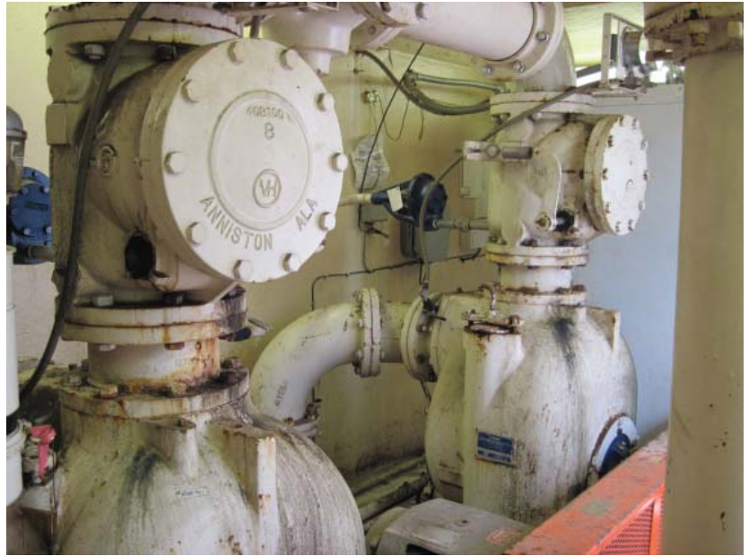
Sewer Lift Station, Fort Benton, Montana
