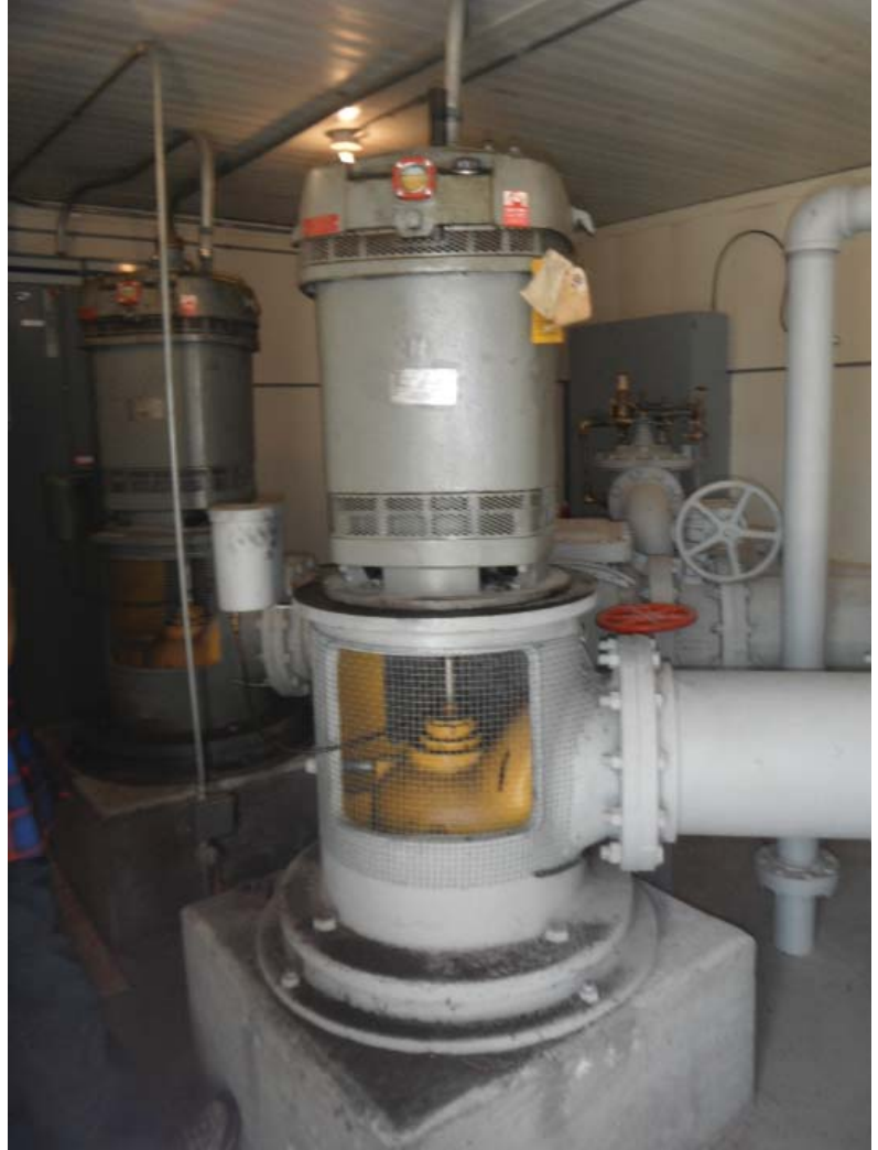
Three Forks, Montana Pump Station
