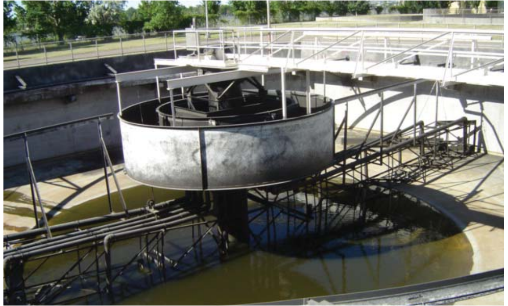
City of Great Falls Wastewater Treatment Plant. Final Clarifier Basin No. 2, emptied for maintenance and examined to design duplicate for new clarifier equipment.
