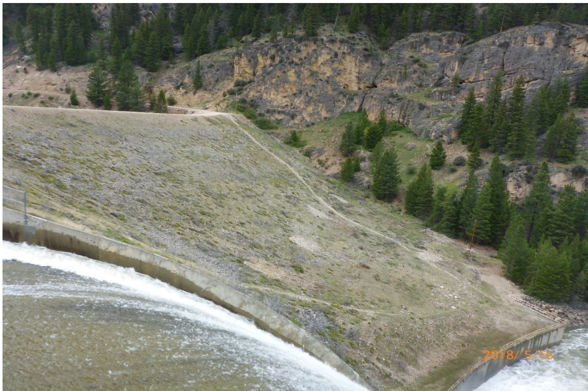
Toe area of Painted Rocks Dam, currently inaccessible by vehicle without fording river.
