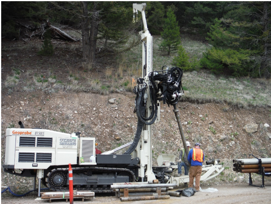
Geotechnical Investigation Drilling at East Fork of Rock Creek Dam (Granite County)
