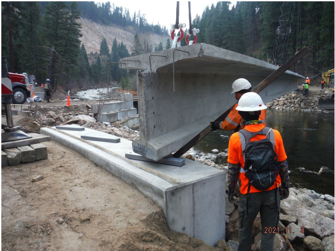
Toe area of Painted Rocks Dam, Setting Bridge Beams for New Access.
