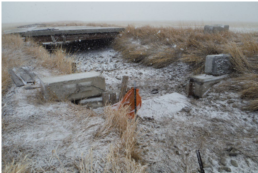
Two Dot Canal – Road Crossing and Check Structure Needing Repairs
