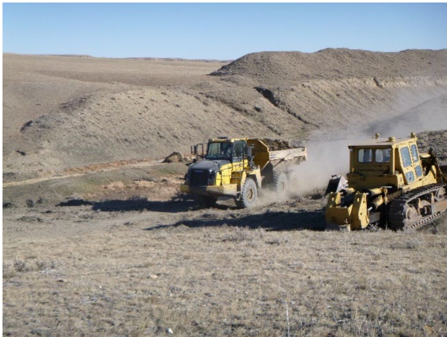
Deadman’s Basin Supply Canal – Transporting Excess Sediment
