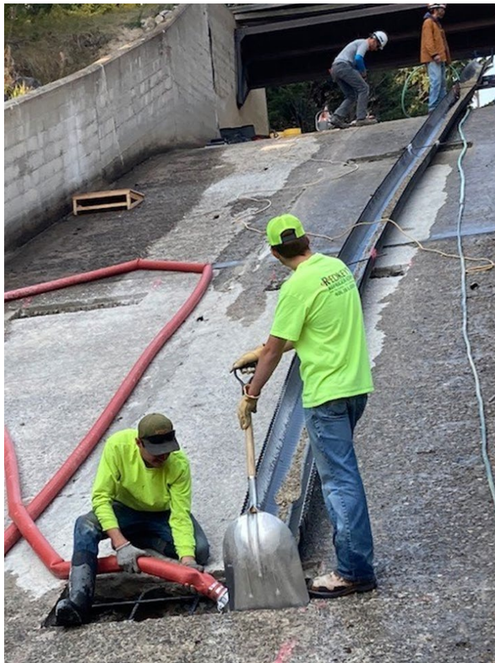
Emergency spillway repairs at Fred Burr Dam after annual inspection discovered voids under the spillway floor.
