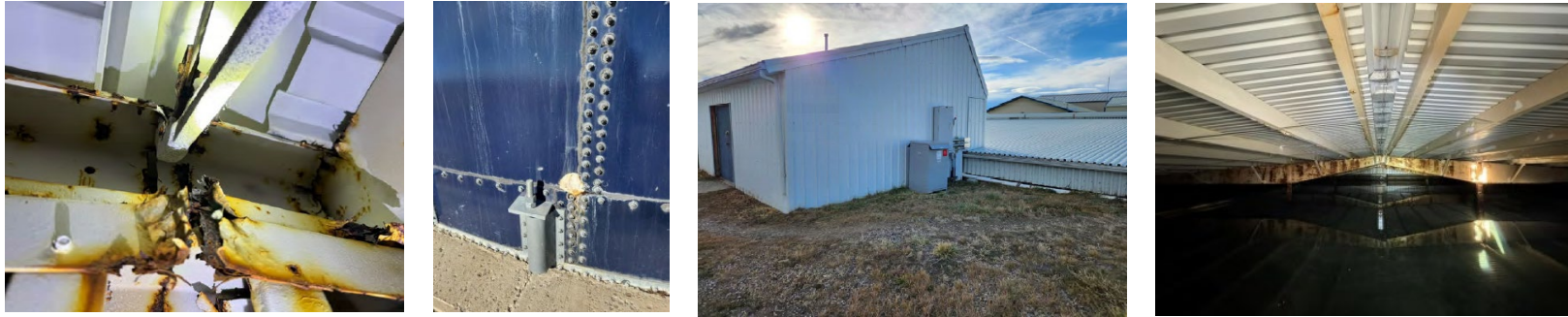
Water system. Photo credit: Sun Prairie Village County Water and Sewer District, 2024.
