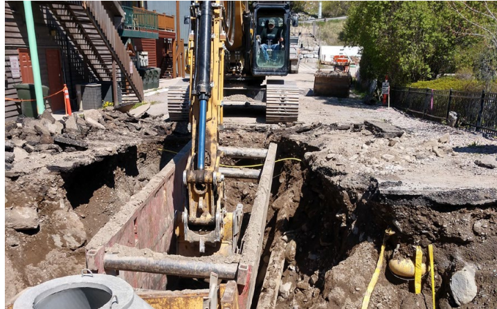
Wastewater system. Photo Credit: Big Fork Water and Sewer District.
