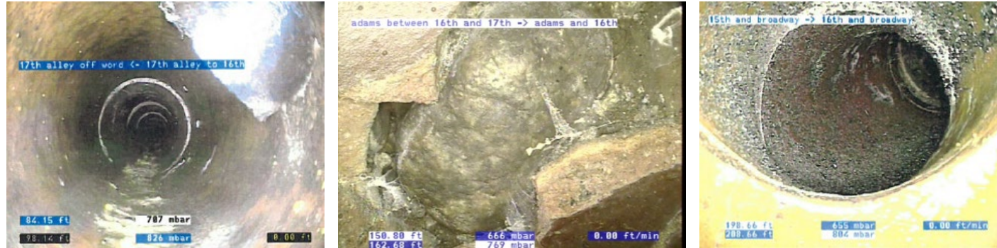
Wastewater system. Photo credit: City of Red Lodge, 2024.
