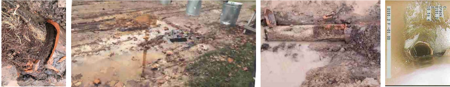
Wastewater system. Photo credit: Town of St. Ignatius, 2024.
