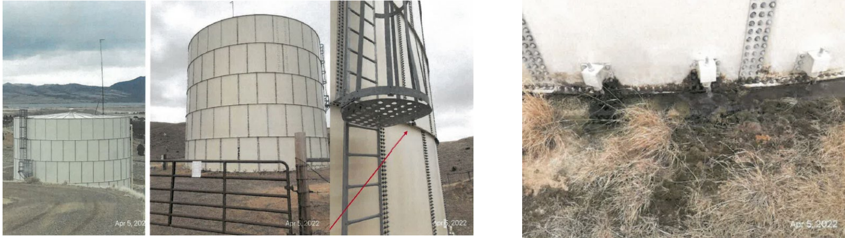
Water system. Photo credit: Town of Ennis, 2024.
