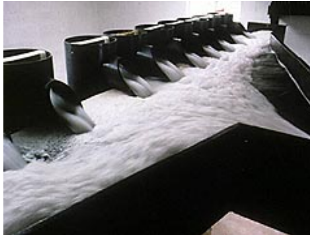
Figure 1-8. In-Line System to Treat Acid Mine Drainage.
