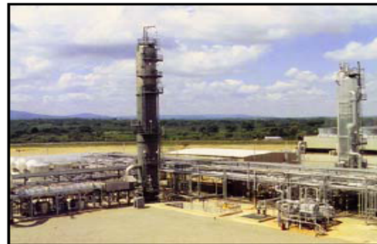
SHADY POINT, OKLAHOMA, USA An AES CFB power plant with MEA CO 2 separation
